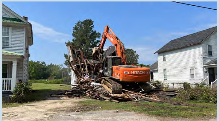
Flippin Construction takes the first swipes of demolition of several dilapidated structures in Lake City. The company won the bid to demolish the six properties in the first phases of blight removal. (Photo by Jonathan Laster)
