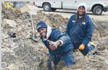
La'Quavion Robertson and Thomas Murrain of Lake City Public Works, do maintenance work on a sewer line on North Matthews Road.
