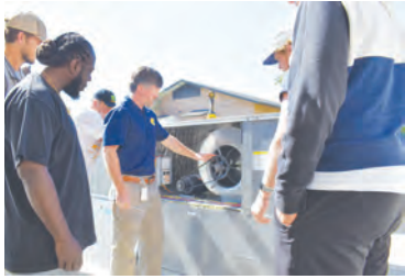
FDTC HVAC Program Director Matthew Lewis instructs his class on a piece of equipment donated by Johnstone Supply
